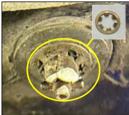
Photo No. 7: Incorrect combination
