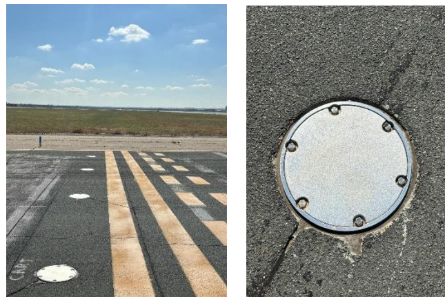
Photographs 5: Holding point signal at E1
